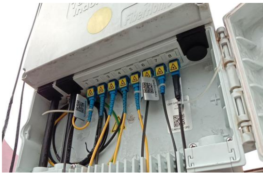
Gambar. 5 Optical Distribution point (ODP)
