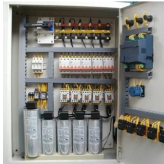
Gbr. 3 Panel Kapasitor Bank
