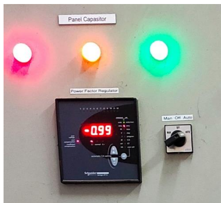
Gbr. 4 Panel Kapasitor Bank
