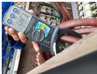
Gbr. 5 Hasil total Arus 16 Fan Main Transformer
