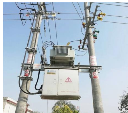
Gambar 2 Transformator Distribusi SM-25kVA-0.69/0.4kV
