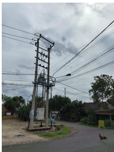
Gbr 4. Gardu Distribusi BH0777
