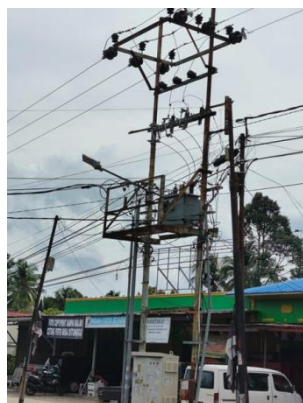
Gbr 2. Gardu Distribusi BH0541
