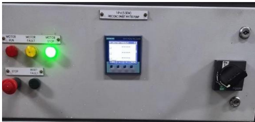
Gambar7. panel control 1-P-6
